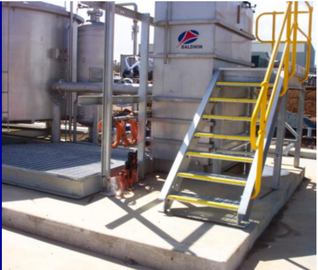
40,000L/Hr PLC Controlled Mine Site DAF
